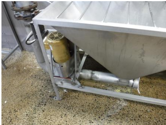
Repair leaks to keep organic material and water contained. Microorganisms require these to survive.
